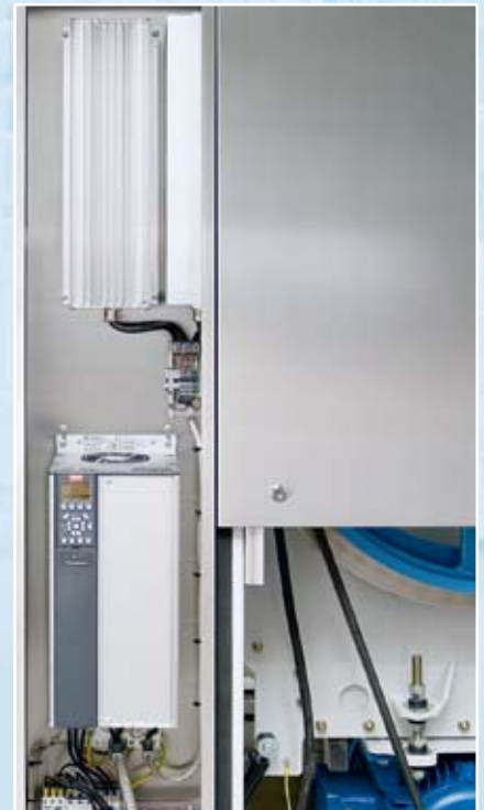
Electrical brake resistors and frequency inverter
